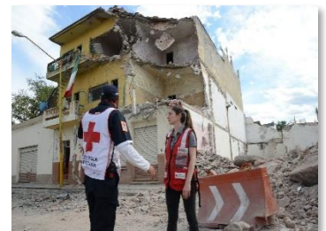
An American Red Cross and Mexican Red Cross team survey damage in a small Mexican city that suffered massive damage when a 7.1 magnitude earthquake struck in 2017.
